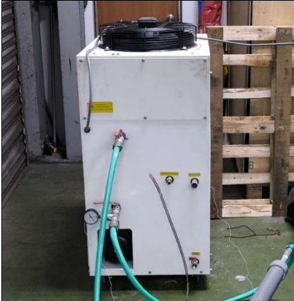
1.5 RT Water-cooled Chiller
