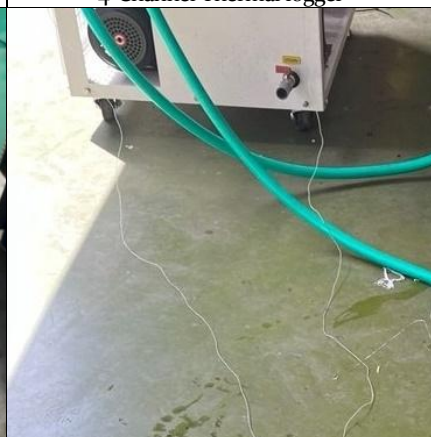
Temperature Sensor at Inlet and Outlet of the Chiller
