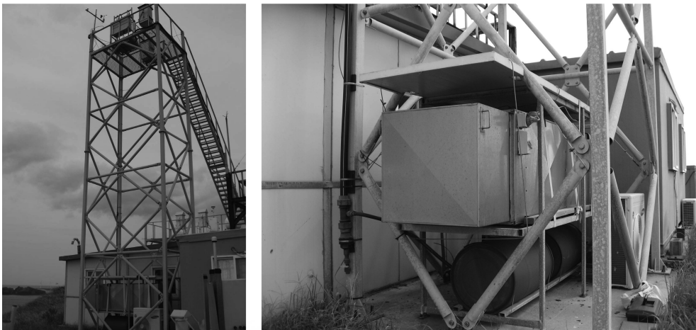
Fig. 3. High sensitivity radon detector system installed at Gosan station of Jeju Island.
