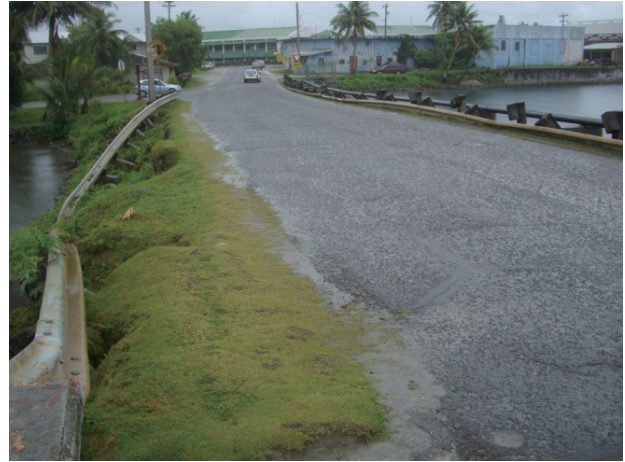
Picture 4. Colonia - devastations around bridge caused by typhoon Sudal.
