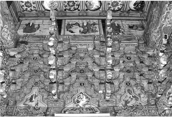
Figure 24. Arhats , detail, the Late Joseon, interior wall of Geungnakjeon of Cheoneunsa Temple, Gurye
