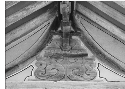
Figure 20. Supporting Plank on the Side Wall of Geungnakjeon Hall, Muwisa Temple (Cultural Heritage Administration 2004)
