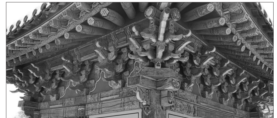
Figure 16. Brackets on the Side and Rear of Josadang Hall, Silleuksa Temple (Photo by the Author)
