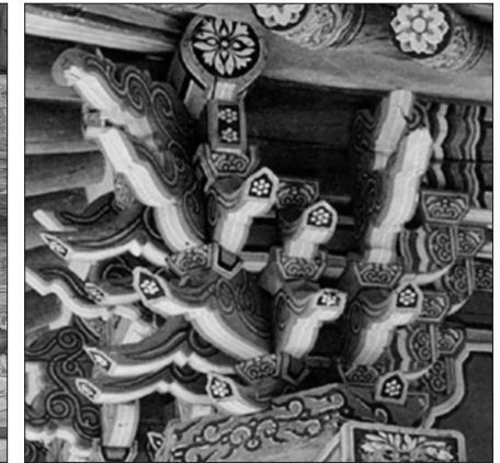
Figure 15. Frontal Corner Bracket of Josadang Hall, Silleuksa Temple (Cultural Heritage Administration 2005b)
